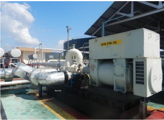
Figure 1. Centrifugal Feed Pump 946-P-1B
