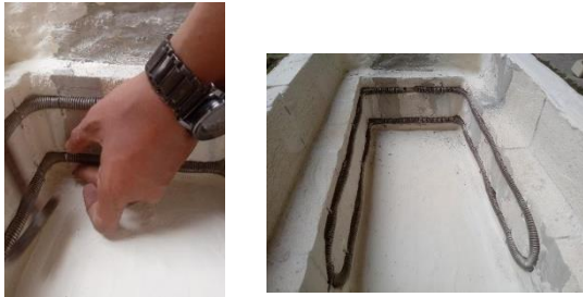
Figure 10. The process of laying the heating coil on the wall of the furnace
